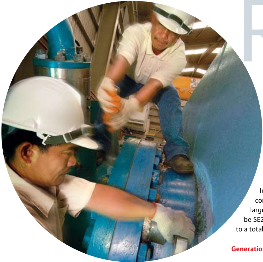
Luzon Hydro personnel conduct a maintenance check on the turbines inside the Bakun AC plant.
